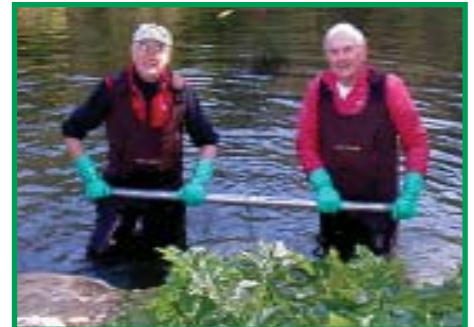
David Bridgham and Fred Ehrman in their waders getting ready to place a concrete base in the pond.
